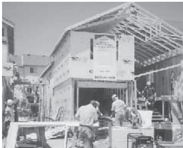
Last June, a number of Habitat houses were built in Waterloo Region. This is a scene from one of the building sites.
