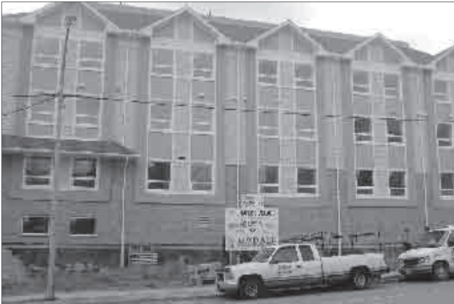
The new Charles Village facility being built by House of Friendship in Kitchener.
