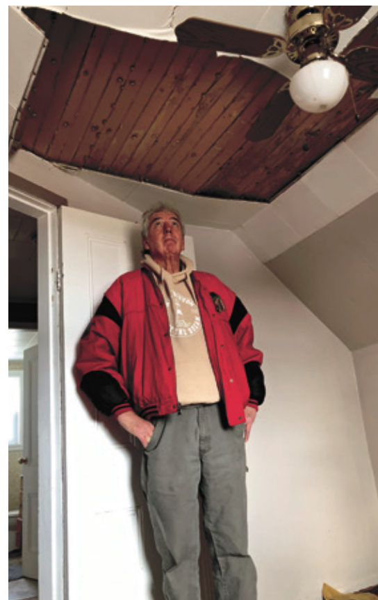
James Towers surveys Hurricane Fiona damage inside his home in Cape Breton.
