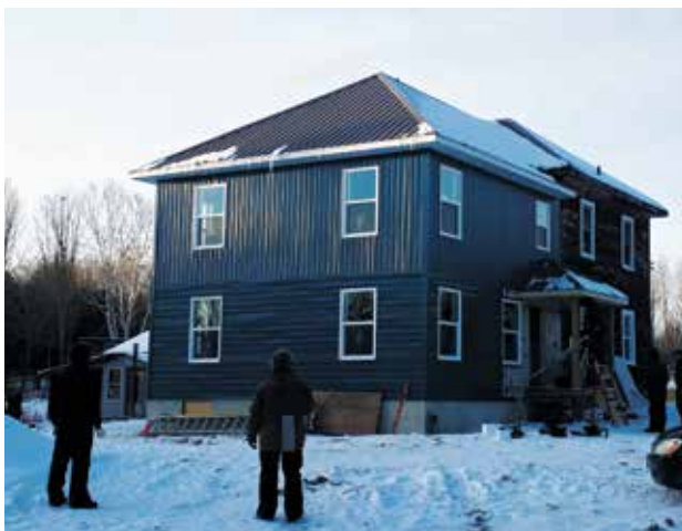
MDS volunteers work on the siding of the addition to the Jobin family’s farmhouse in Barry’s Bay, Ont.
