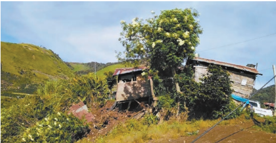
A home destroyed by the late October earthquakes on the island of Mindanao.
