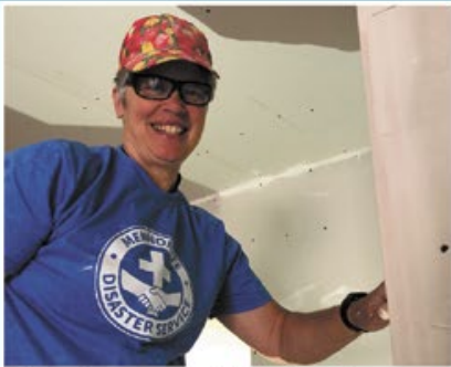
Jan Joyce working in a home in Grand Forks, B.C., damaged by the 2018 flood.
