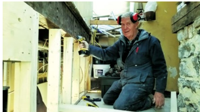
Peter Kroeker, a Mennonite Disaster Service volunteer from Vineland (Ont.) United Mennonite Church, works on the exit stairs during renovations at Hochma Mennonite Church to bring its basement homeless shelter up to code.
