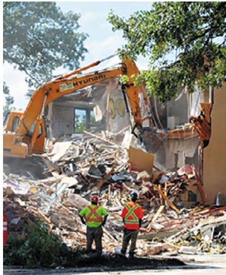
The middle section of Westgate Mennonite Collegiate being demolished in the summer of 2016.
