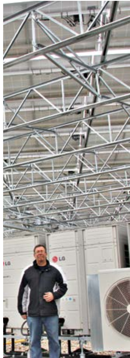
Bob Lebold, 50 Kent Avenue's physical services coordinator, stands in front of the air-to-air heat exchange units on the roof of the building and under the 200-kilowatt solar electric installation.
