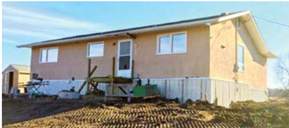
John and Mary Webb’s house nears completion after more than 3,000 hours of repairs by Mennonite Disaster Service volunteers following a 2011 flood of the Red River near Selkirk, Man.
