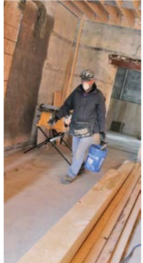
Dan Ulrich of Mennonite Disaster Service works on the Kitchener fire rebuild.
