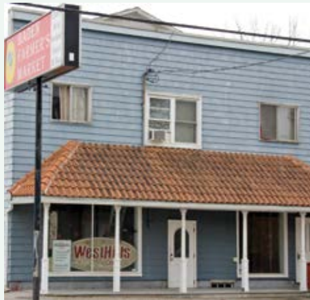
West Hills Mennonite Church is converting the Baden Emporium building in Baden, Ont., into its new church and community space.
