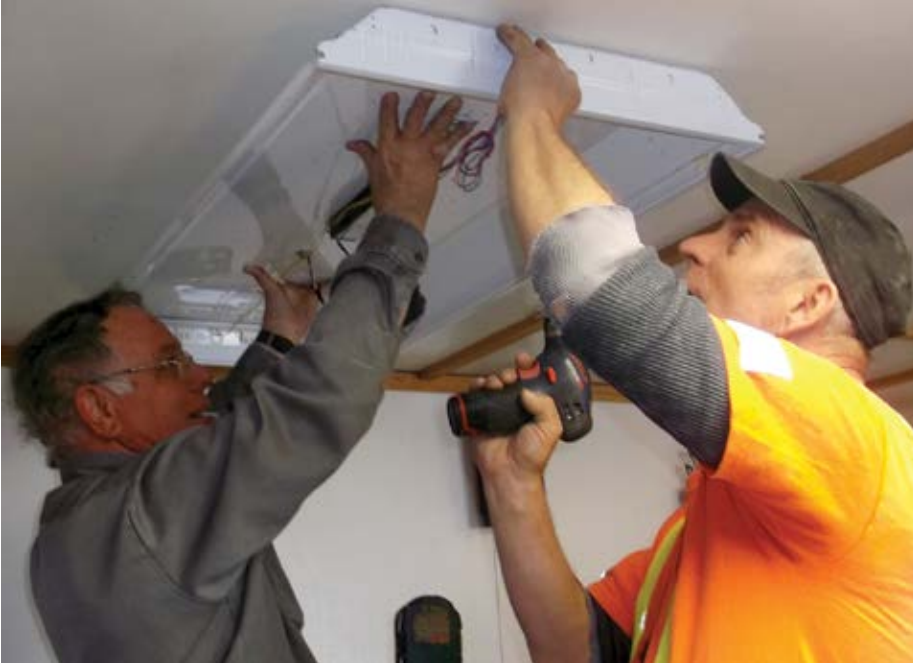
Larry Bearss, left, and Mike Henderson replace light fixtures on the Attawapiskat First Nation as part of a joint MCC Ontario/Mennonite Disaster Service initiative that also involved Ontario Power Generation and the Mushkegowuk Council.
