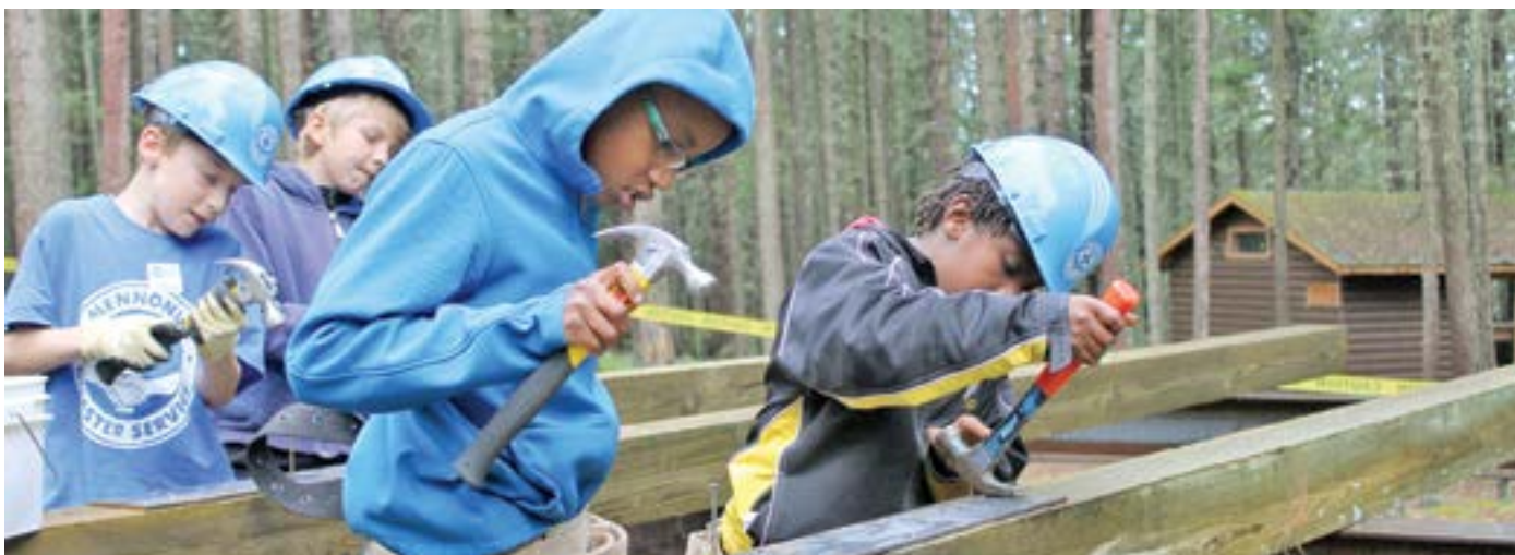
Samuel Friesen, left, Levi Jowett-Stark, Kobe Friesen and Asher Warkentin are hard at work pounding nails for the foundation of a new cabin at Camp Valaqua.
