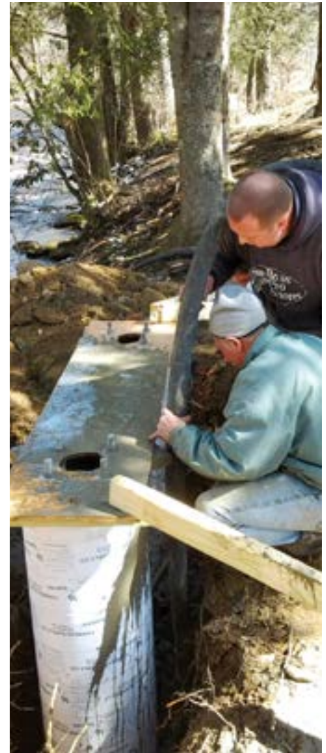
MDS volunteers construct the footers for a new swinging bridge that provides safe passage between the home of Josephine and Garcie Cogar and their community of Webster Springs, W.V. The original bridge was washed out during Hurricane Sandy in 2012.
