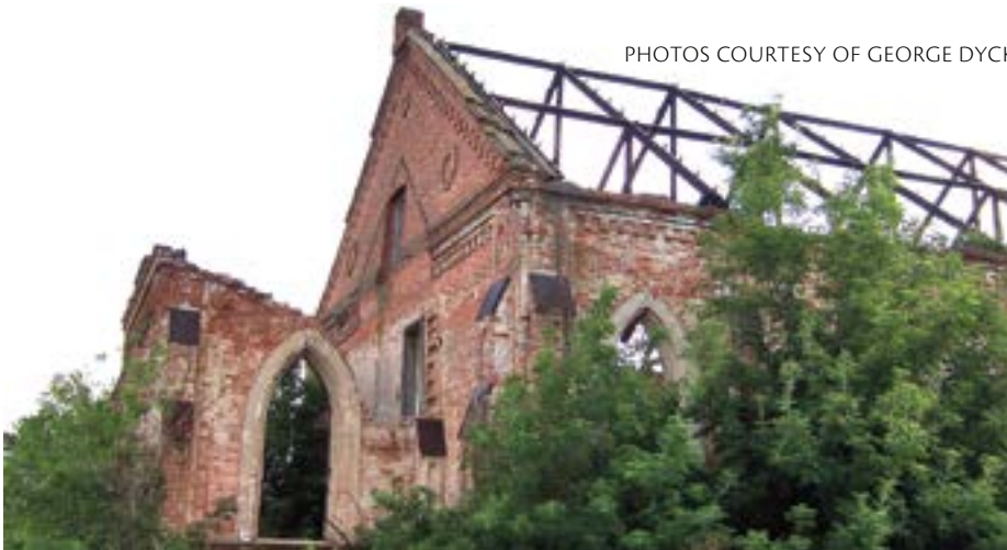
Exterior roof repairs to the former Mennonite church in the former village of Schoensee—now Snegurovka—are visible.
