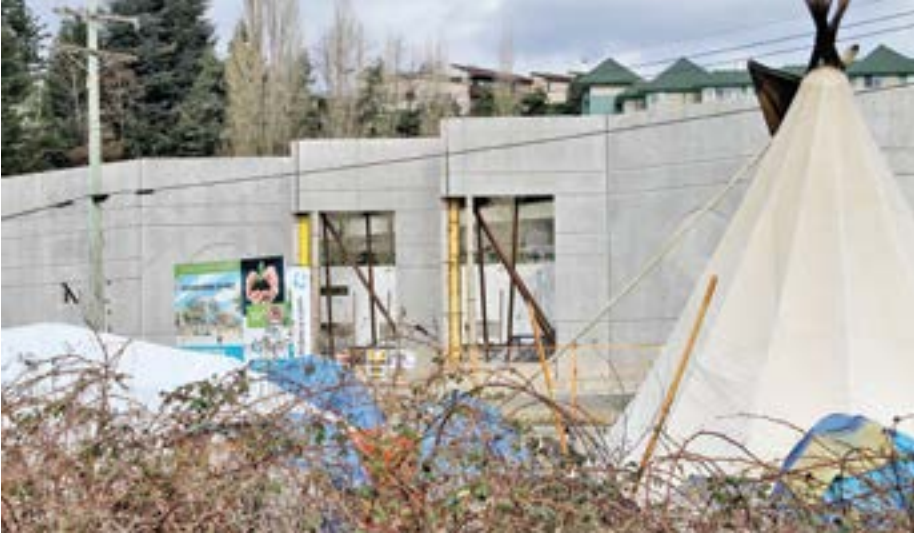
With the new MCC Centre under construction across Gladys Street, a tent city stands as testimony to the problem of homelessness in Abbotsford, B.C.
