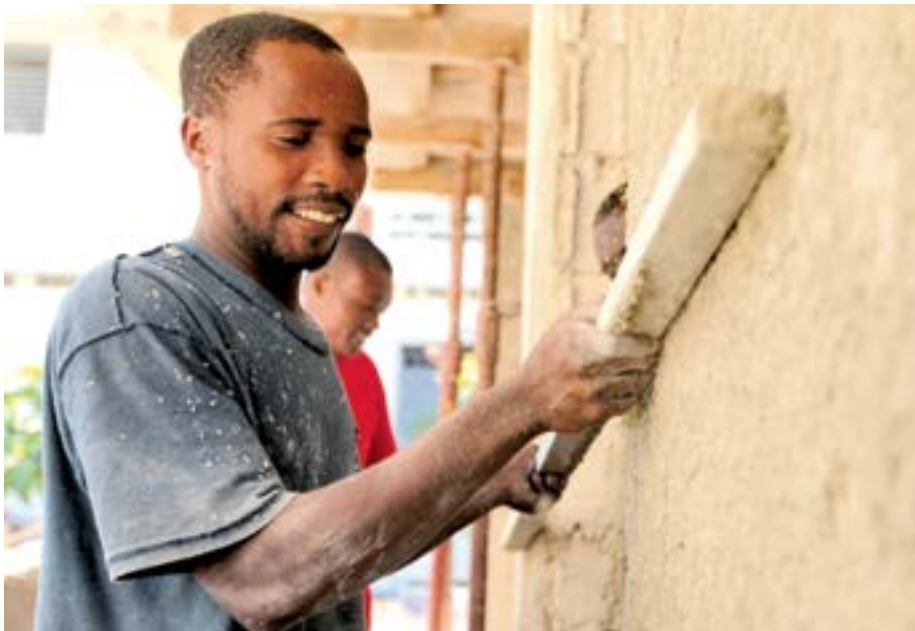
Masonry students such as 25-year-old Ronald Sadou Zami benefited from a 2012 MCC seminar on disaster-resistant construction.
