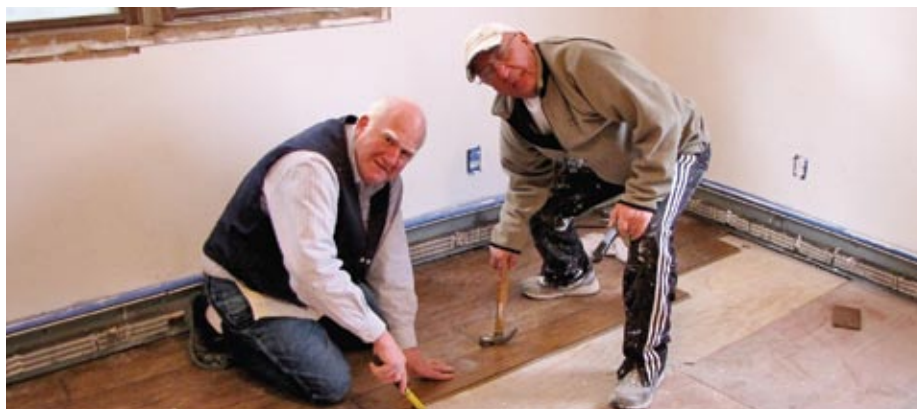
Ivan Martin of New York, left, and Errol Stein of Ontario install new flooring.
