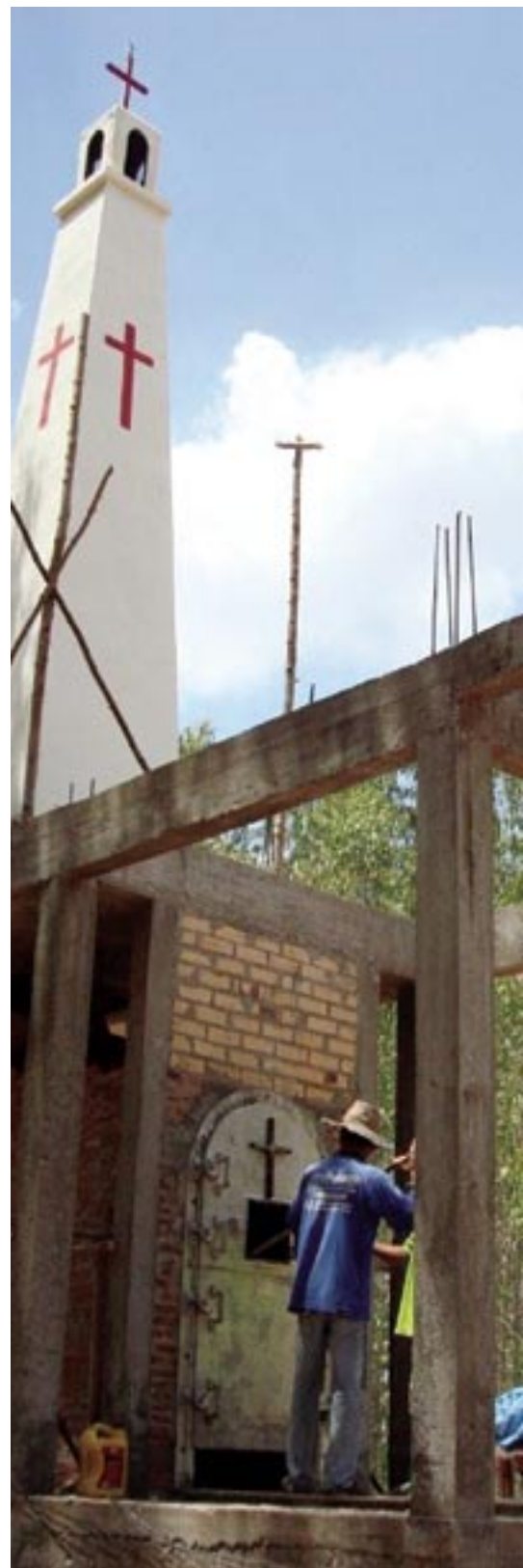
The construction of the crematorium at Living Water Church, Borabu, Thailand, began in February and was finished in June.
