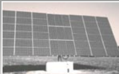
Ground-mount SUNtracker systems
