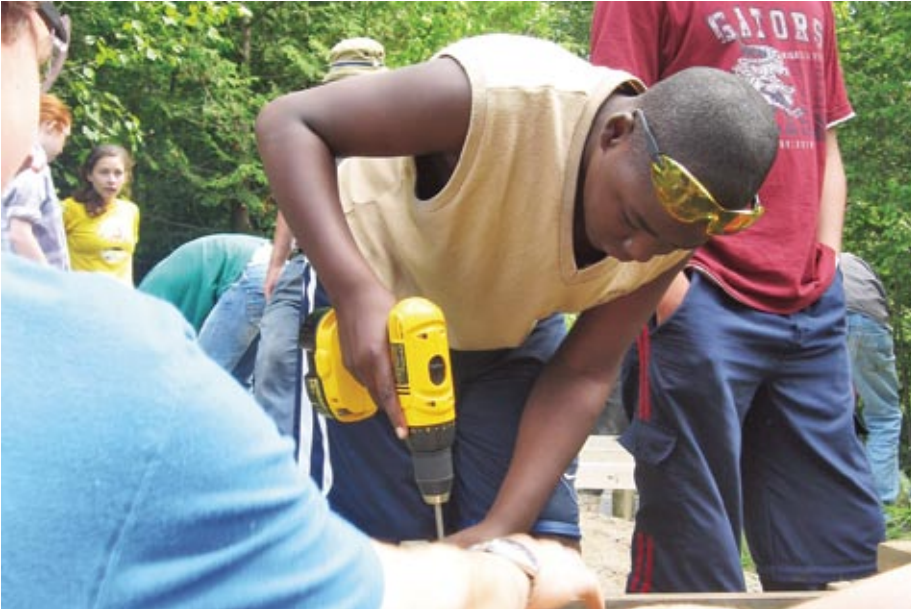
'Kingdom spirituality' is well suited to Mennonites. This is the 'give me something to do for God' spirituality that goes on peace marches, works with Mennonite Disaster Service, sits at the quilting frame or helps with building projects like the one at Silver Lake Mennonite Camp, Ont., pictured.
