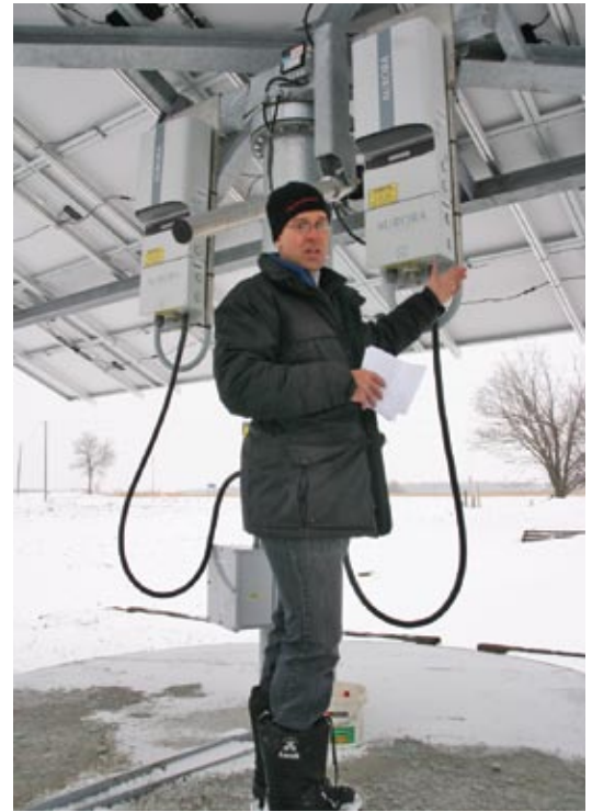
Rob Yost of Hillcrest Mennonite Church stands at the base of the congregation's one-kWh photovoltaic solar-energy system.
