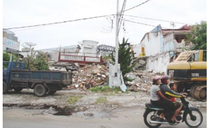
Large machinery is staged in Padang, Indonesia, ready to begin removal of rubble after heavy earthquake damage on Sept. 30 and Oct. 1. MCC representatives are also in Padang, assessing how MCC can be most helpful.
