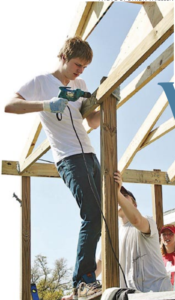
MDS volunteer Mark Heinrichs from Foothills Mennonite Church, Calgary, helps rebuild a home in Cameron, La.
