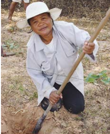
Bualean Bootbangyang digs a hole to help build a fence for Living Water Church in Borabu, Thailand.
