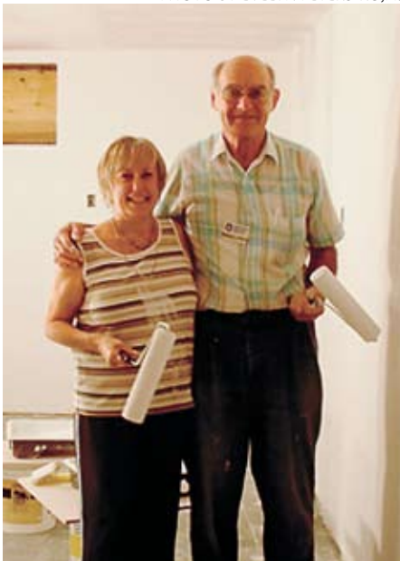
MDS client Trudy Mogg works alongside volunteer George Ediger to prim the walls of her house which suffered flood damage.
