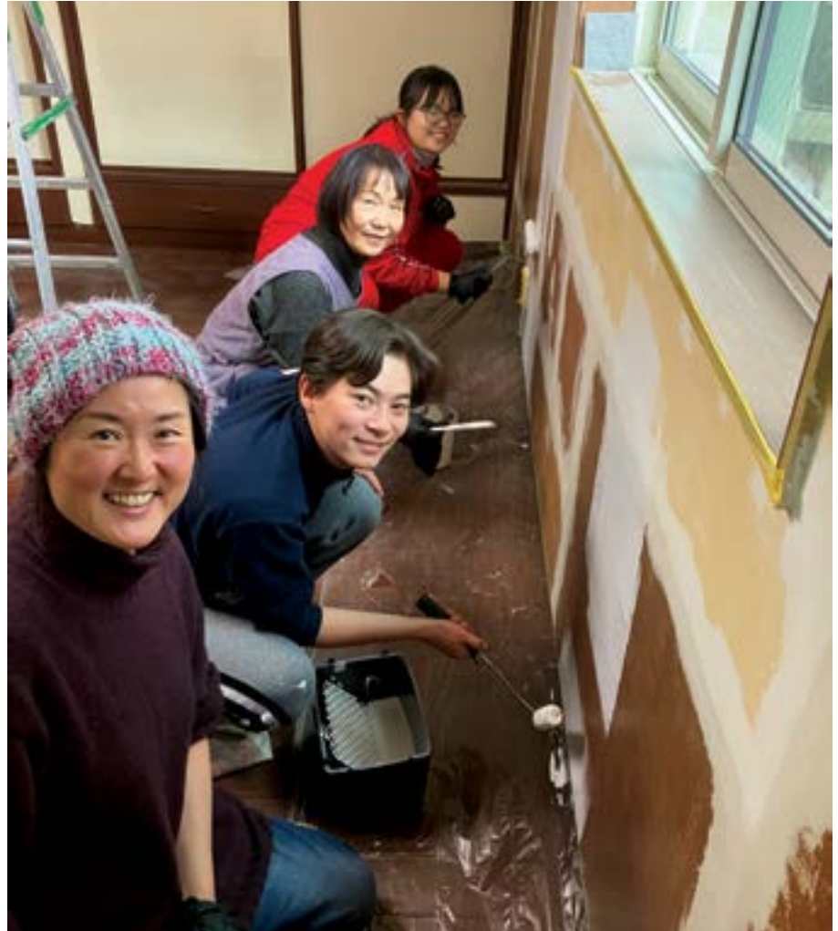
Volunteers prime a wall as part of renovations to the Tokyo Anabaptist Centre. .
